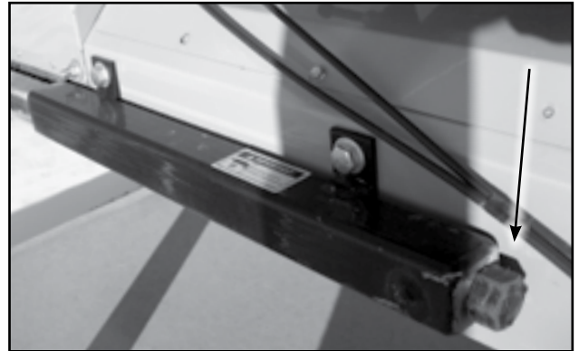
Fig 46 - Conveyor belt tensioning jacks
